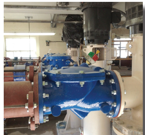
Crystal Springs Pump Station Roanoke, VA
