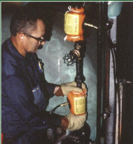
QWIK-FREEZER™ IS USED TO MAKE A DOUBLE FREEZE ON A PIPE IN ORDER TO ISOLATE A VALVE.
