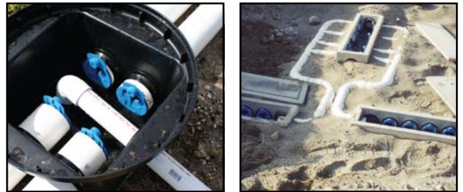
Custom Distribution Boxes with Equalizers installed
