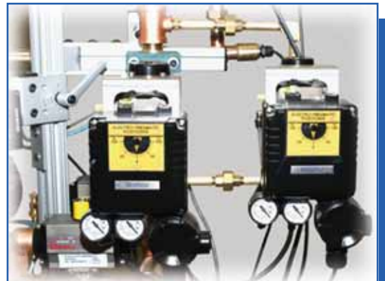
Outlet assembly containing flow control valves and flow transmitter
