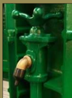
Protective Caps On All Outlets
